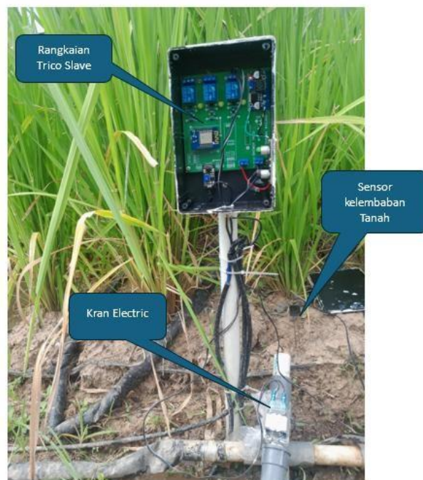
Figure 5. Trico Master and Slave Installation in the Field
